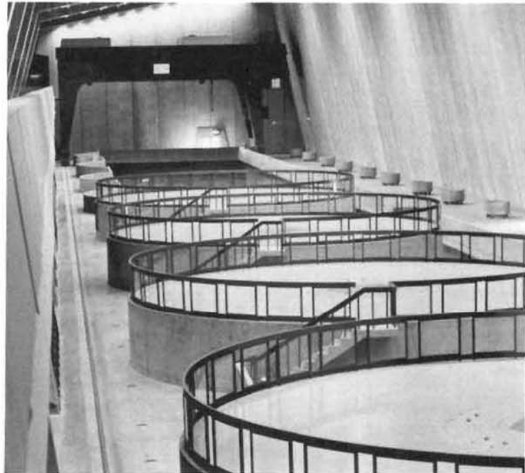
POWERHOUSE INTERIOR at Libby Dam.
