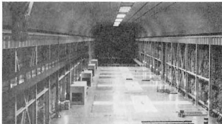
UNDERGROUND POWERHOUSE, deck over the generators, at Mica Dam.
