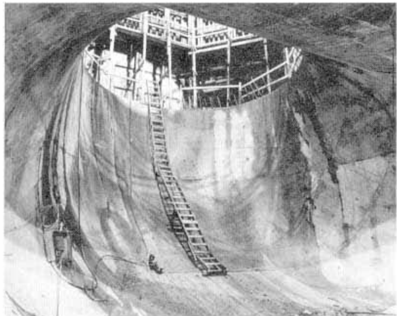
DRAFT TUBE ELBOW for Unit No. 1 at Mica powerhouse.
